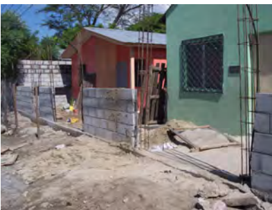
Beginning stages of building the security wall to protect 3 of the 4 buildings where FEVIVA operates
