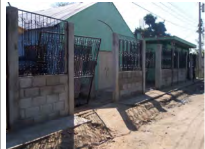
The final stages of the security wall which will afford protection for the activities of God's program
